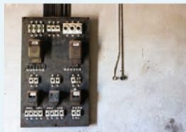
Electrical Switchboard Panels
